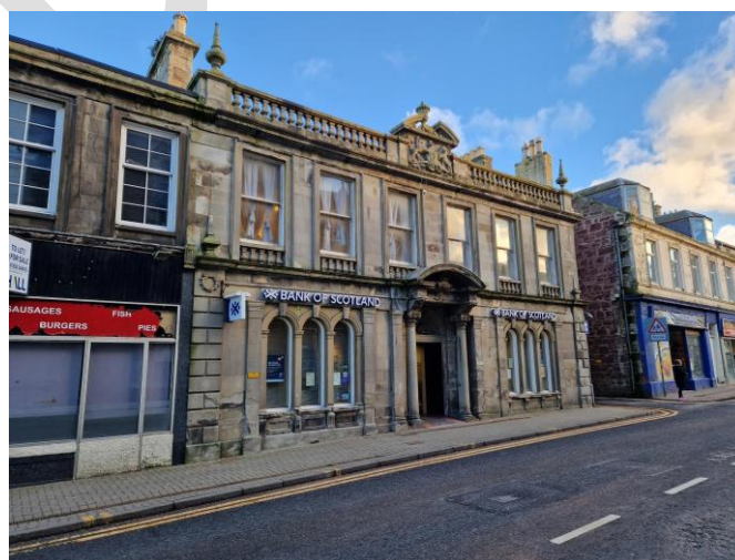
Stonework Erosion, 17 Dalrymple Street
