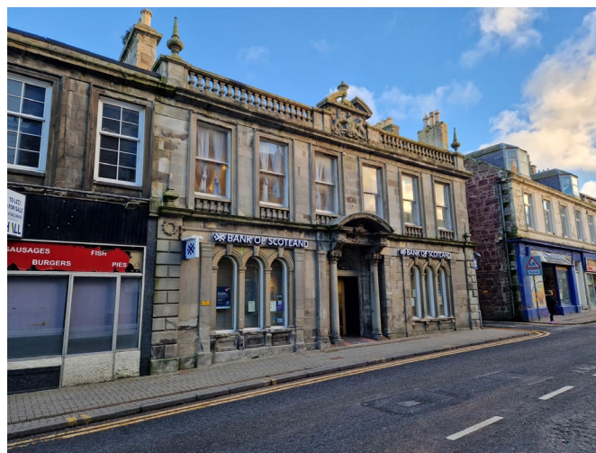
Stonework Erosion, 17 Dalrymple Street
