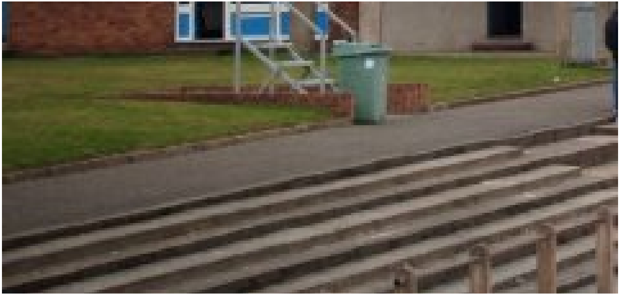
Photograph shows the concrete stepped area referred to in the LSO report
